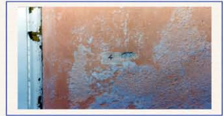
Figure 3 - Detail of marmorino walls at ground floor of Sala Apollinea with deep degradation for saline efflorescence
