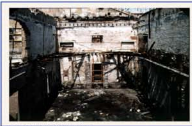
Figure 2 - Same room after devastating fire
